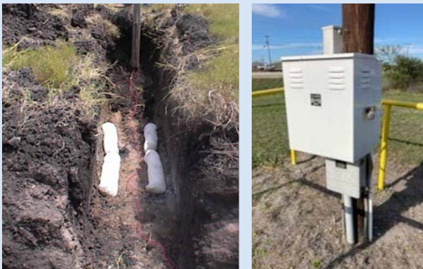
On the right is a photo of one of two rectifiers protecting the 42" line with an impressed current. On the left, is a typical installation of sacrificial anodes on the 42" waterline. Currently, there are two Cathodic Protection Techs installing anodes, adding test stations and, in general, upgrading the 42" waterline using remaining 2012 bond funds.
