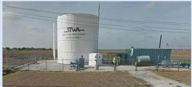
Agua Dulce Pump Station, used by both the City of Agua Dulce and Nueces Water Supply Corporation.
