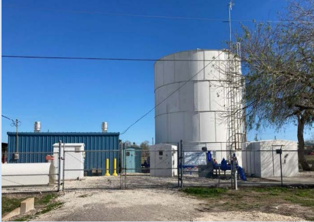
Driscoll Pump Station, which serves City of Driscoll and Nueces WSC customers.
