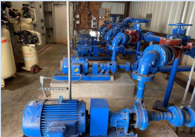
Central Pump Station interior (provides water to NWSC rural customers and also boosts pressure to Agua Dulce, Banquete, and Sablatura Park Pump Stations).
